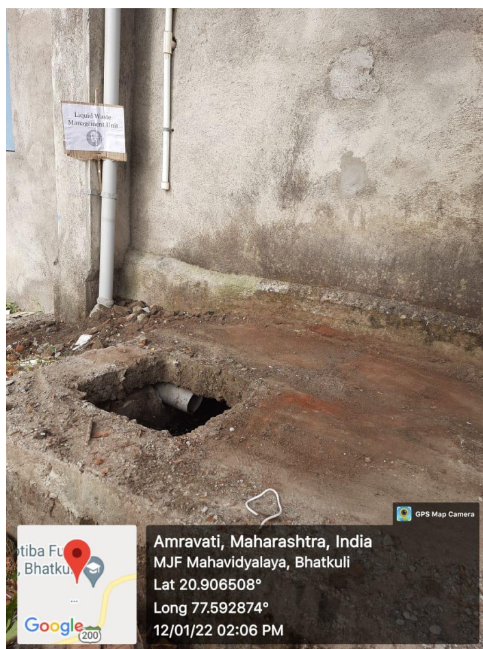
Liquid Waste Management Unit
